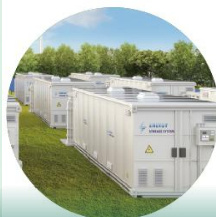
CO detector for BESS
