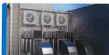
Central air conditioner
